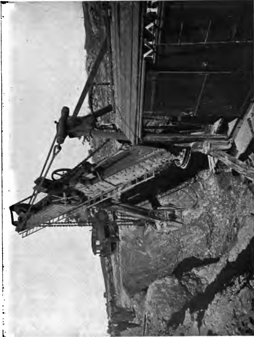
PLATE 131. —Special 90-ton Marion Steam Shovel with Long Boom. Lift 26 feet, cast 35 feet. This shovel excavated full depth of cut to close lines and filled cars on banks which were dumped over completed aqueduct. Machines similar to this were extensively used on Catskill Aqueduct construction.
